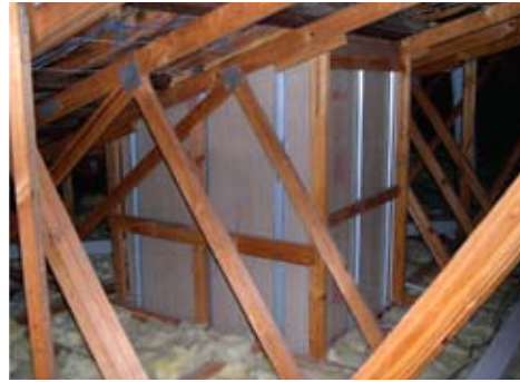
Roof framing: plantation softwood. Note the skylight shaft to the family room.
