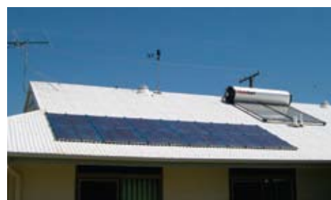
Two arrays of PV cells and the solar H/W unit.
