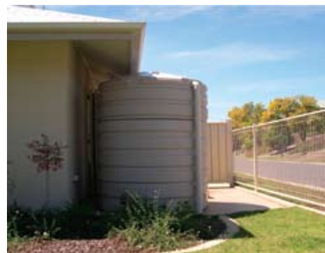
The 2kL rainwater tank at the S/E corner.
