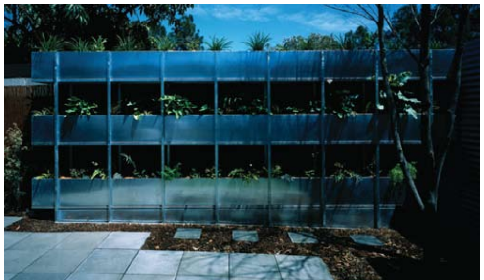
This vertical greywater filtering system treats water to be re-used in the toilet, washing machine and garden.
