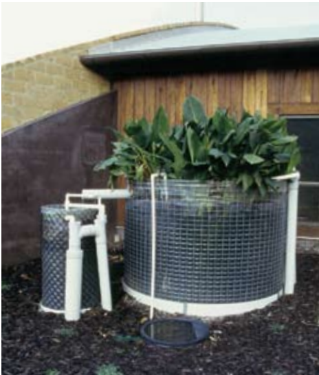
On-site sewage treatment system.
