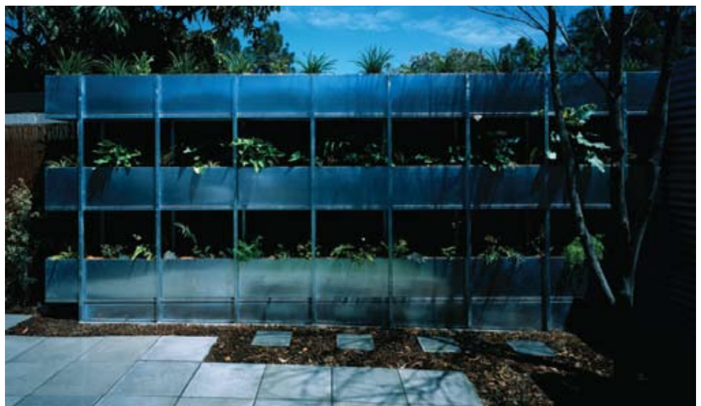
This vertical greywater filtering system treats water to be re-used in the toilet, washing machine and garden.
