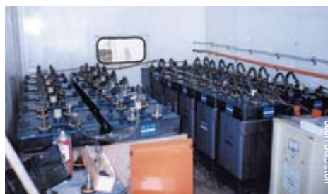
A battery bank.
