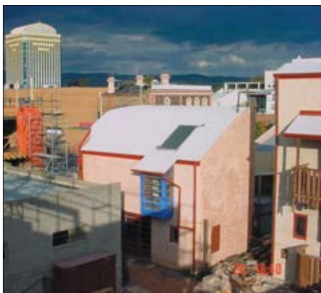
Straw bales in the city. There is no location that straw bale building cannot adapt to.
