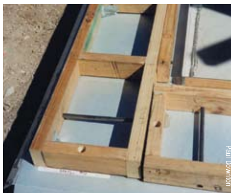
Ladder frame bottom compression plates being bolted to concrete slab through ant-cap damp course showing recycled irrigation hose for sleeving high tensile wire through pea gravel base.
