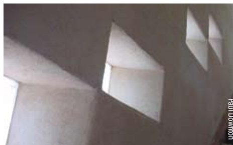
This dry-lined interior shows how AAC can be exploited to make niches and unusual openings.
