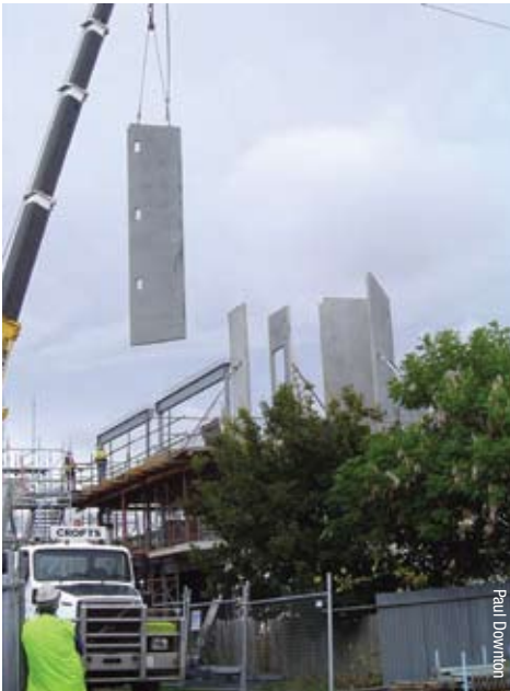
Dense precast concrete panels provide structural support and appropriately located thermal mass for this five storey apartment building, seen here under construction.
