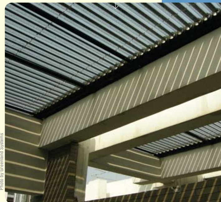
These evacuated solar thermal tubes powered the airconditioning at the Beijing Athlete's Village
